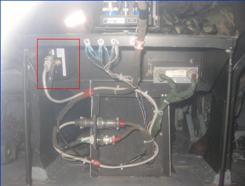
Location of AK-550 altimeter at the central console in the cockpit of Mi-8T RA-24105 and RA-24125 helicopters (looking aft).
